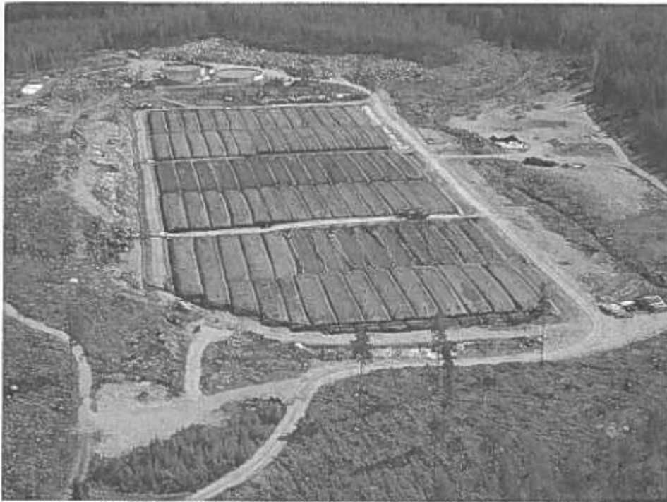
Fig. 5: Aerial view on the landfill site with the filled geotubes. The water treatment plant can be seen in the back.
